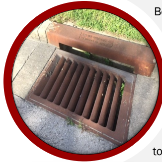
Water flows into these catch basins and straight into our waterways!
