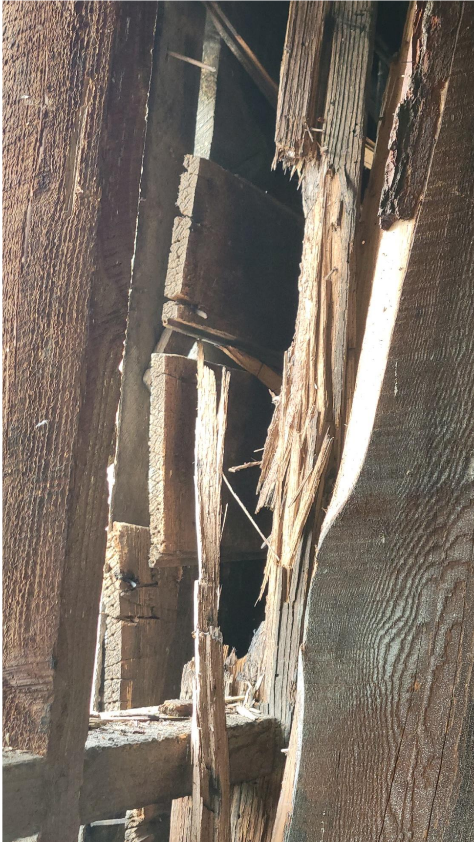
Photo 11: Interior wood shredded in belfry and charred. (It's amazing no fire started!)
