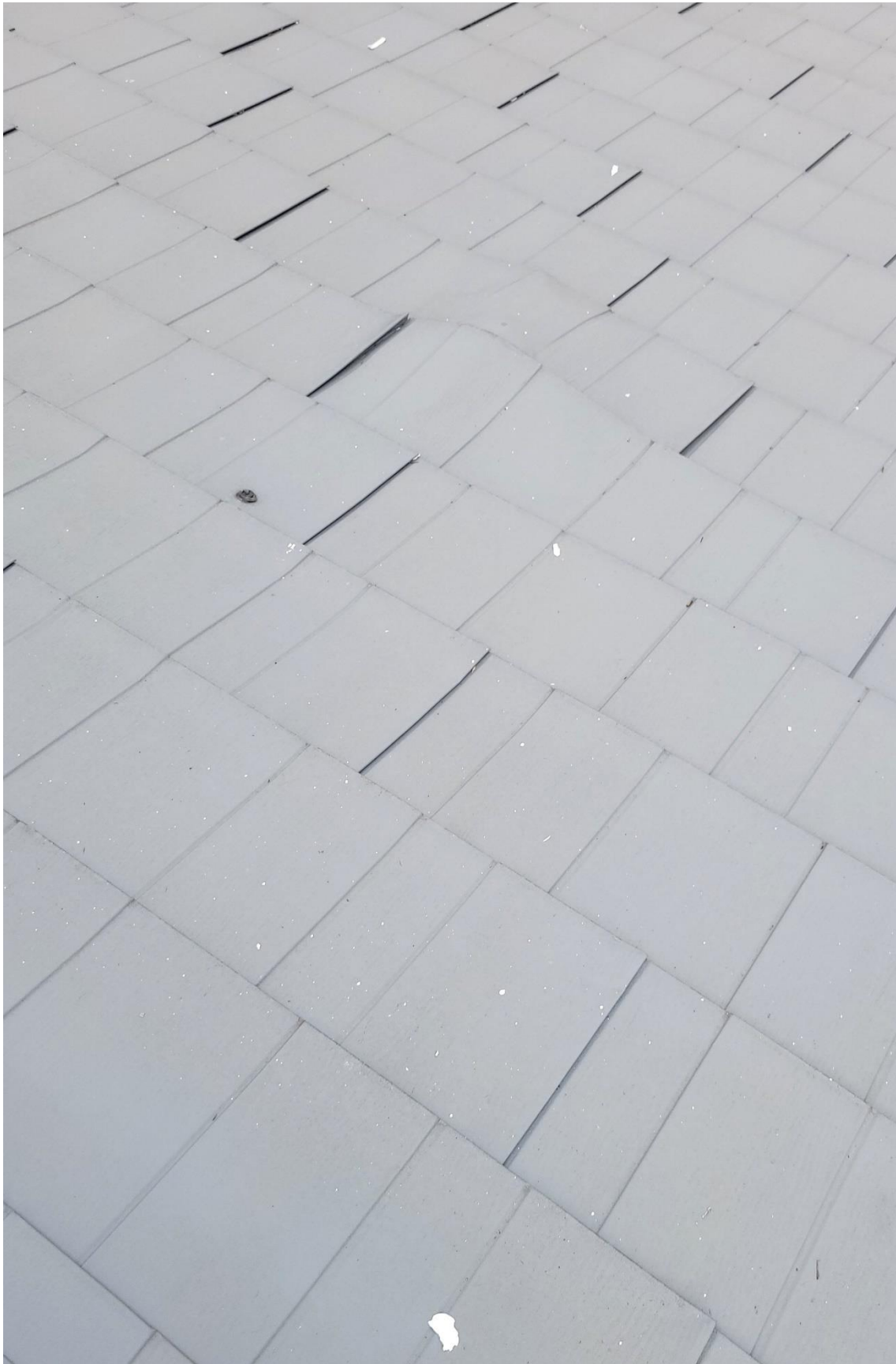
Photo 14: Closeup of roof tiles showing pattern. Note ripple in center caused by force of lightning,
