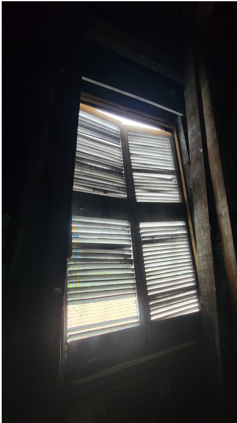
Photo 3: View of damage to shutters
