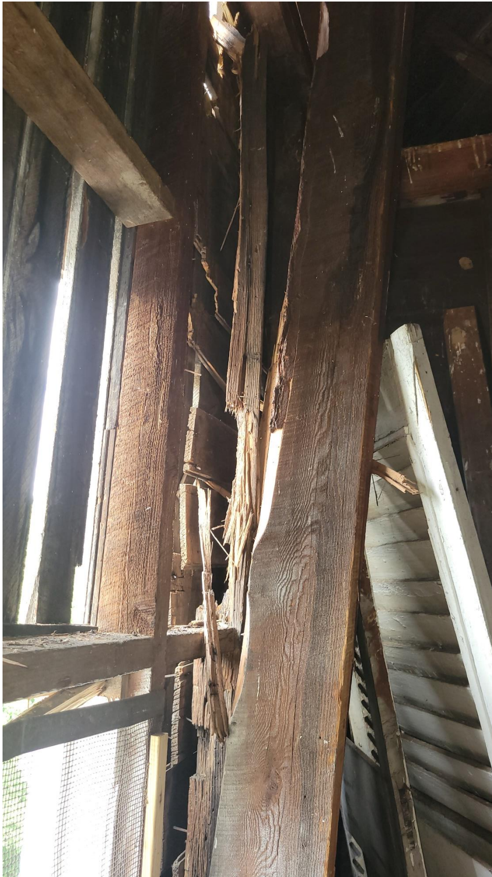
Photo 9: Interior structural damage in belfry
