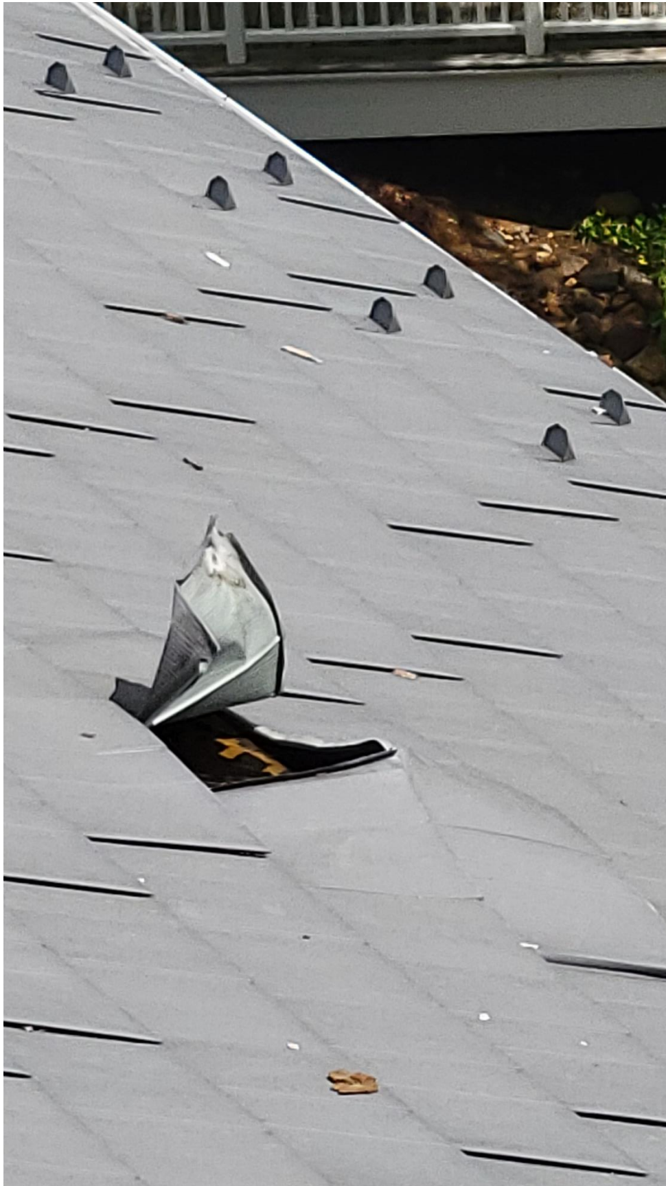
Photo 12: View of damaged tin roof tiles. We believe this is where the lightning exited
