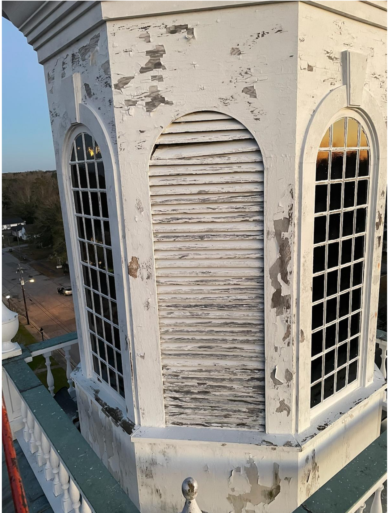
Photo 6: Shutter in similar state of deterioration as ours are currently
