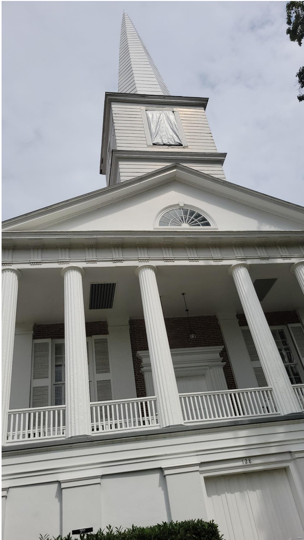
Photo 5: View of where south shutter was prior to August 14 storm that destroyed that shutter
