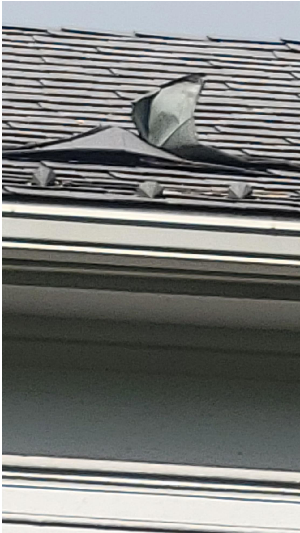
Photo 13: Another angle of roof damage, the existing painted tin roof was installed in 2003 and is beginning to rust
